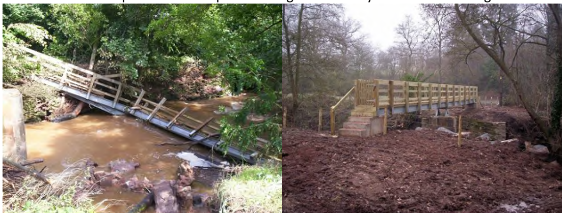
Before and after photo of the Papermill Bridge in Cleobury Mortimer – damage due to flooding!
