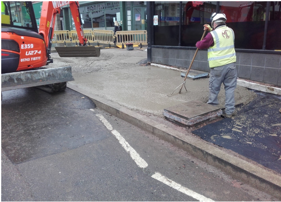
Placing concrete sub base layer prior to laying yorkstone slabs at Barker Street / Claremont Hill junction
