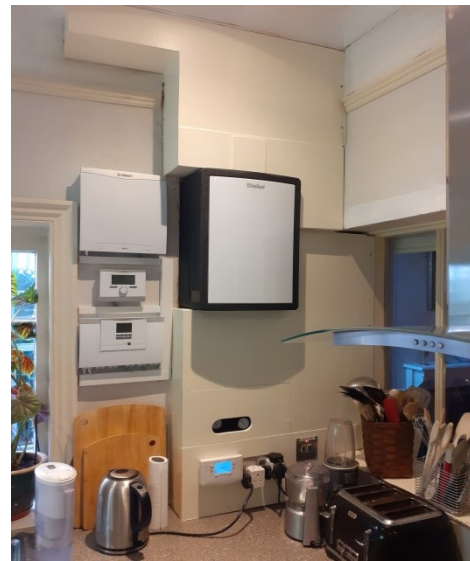
Heat exchanger and controls where the boiler used to be.
