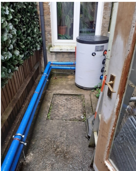
Tank now sits in a waterproof extra insulation box.
