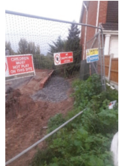
Figure 21 – Developer blocking a footpath in Shrewsbury
