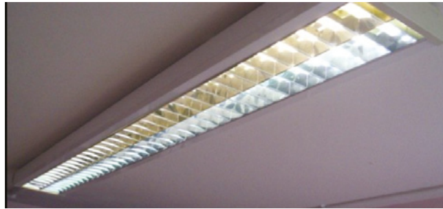
Figure 28: Poor maintenance illustrated by mixture of lamps in luminaire
