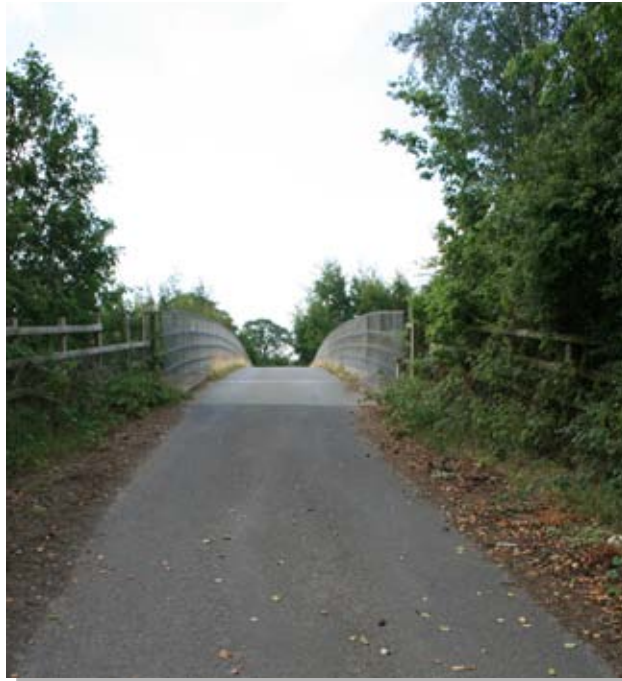
A5(T) overbridge provides a public link between the site and the countryside to the south.
