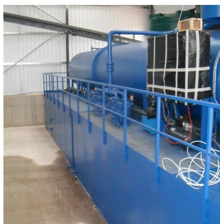
Figure 8: Tanalith E storage tanks containment bunds Visible water is from rain prior to building erection
