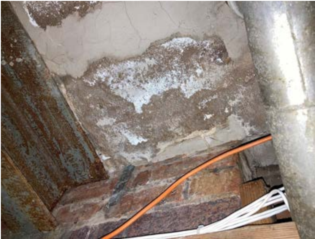
Photograph 2 water ingress and efflorescence.
