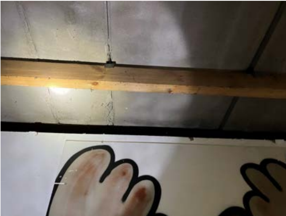
Photograph 13 typical panel damage at edges and bearings.
