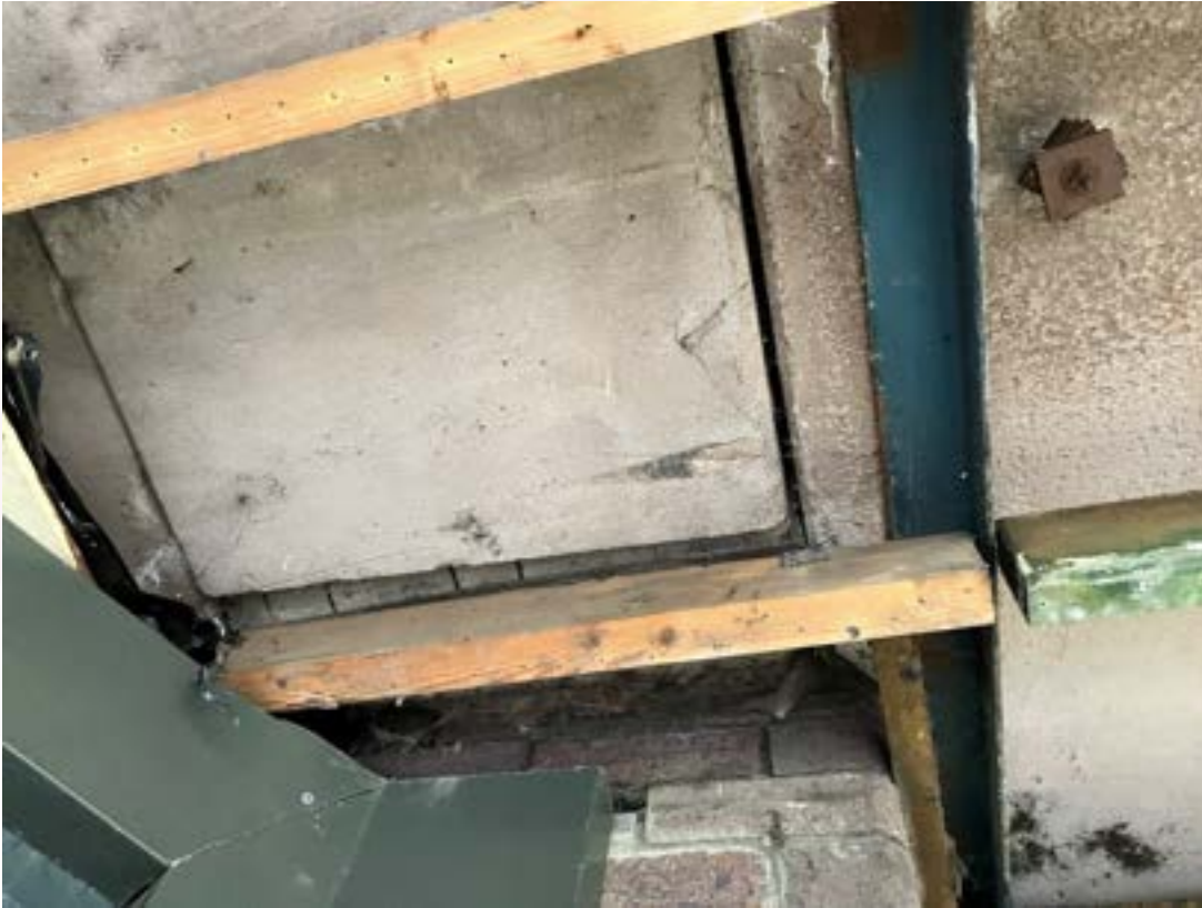
Photograph 12 cut panels poorly supported and exposed reinforcement also displacement between adjacent panels.
