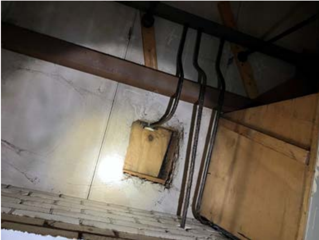
Photograph 14 unsupported large opening to panels ground floor rear rooms at back of stage.
