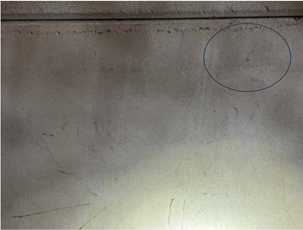
Photograph 19 hairline cracking to panel.
