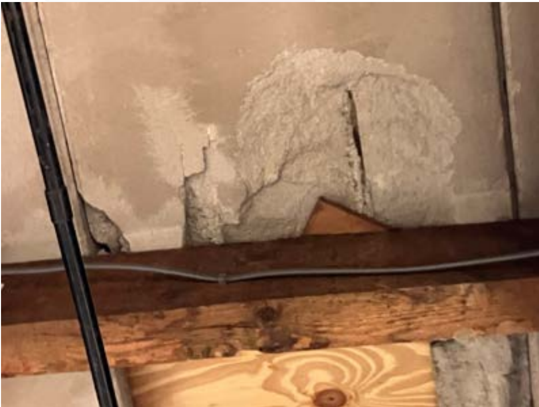
Photograph 7 damaged panel adjacent to a cut opening with additional support from timber joist.
