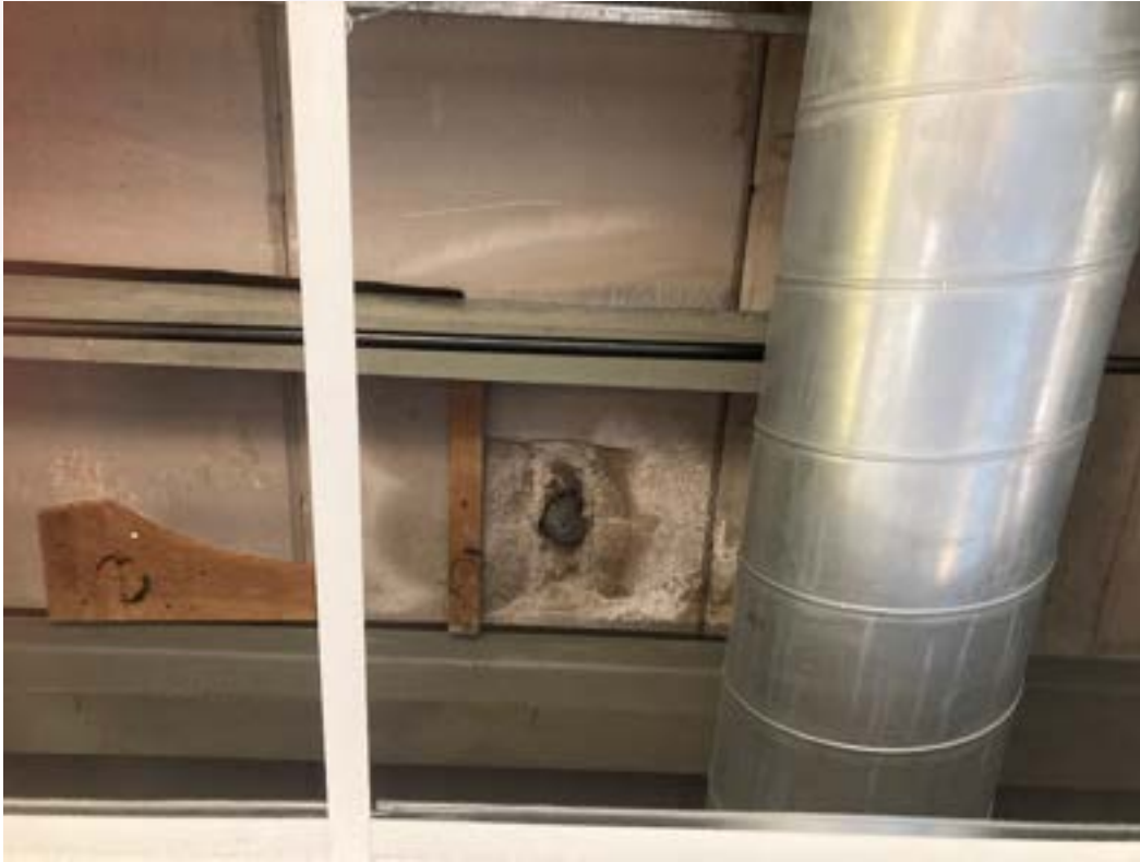
Photograph 1 RAAC panel with hole filled with wire wool and further damage and water ingress.
