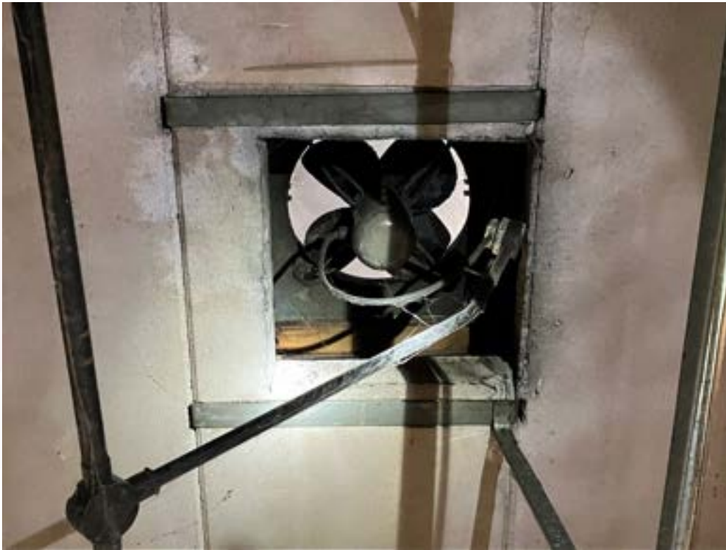
Photograph 4 typical fan installation with damaged cut ends and proprietary supports.
