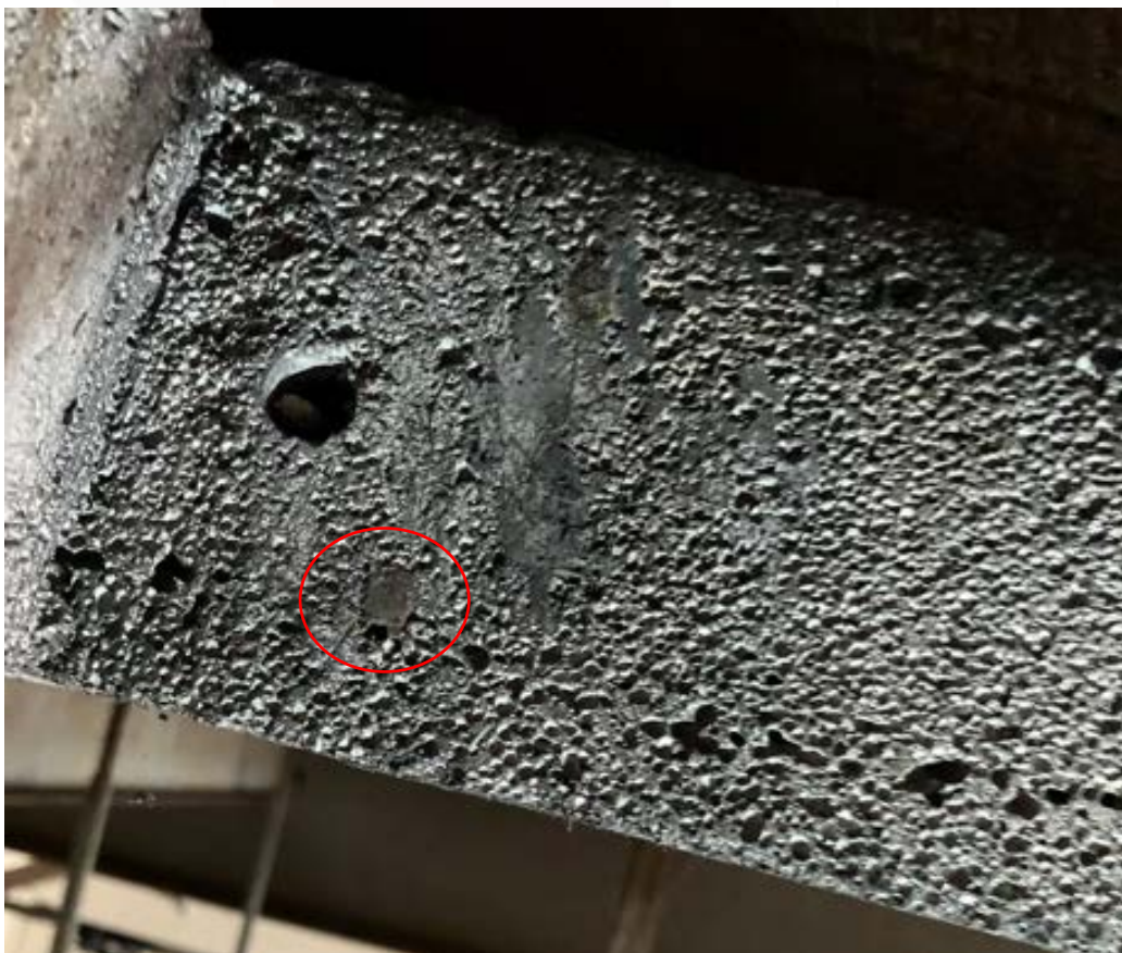
Photograph 5 single transverse reinforcement bar in fan opening and large void.
