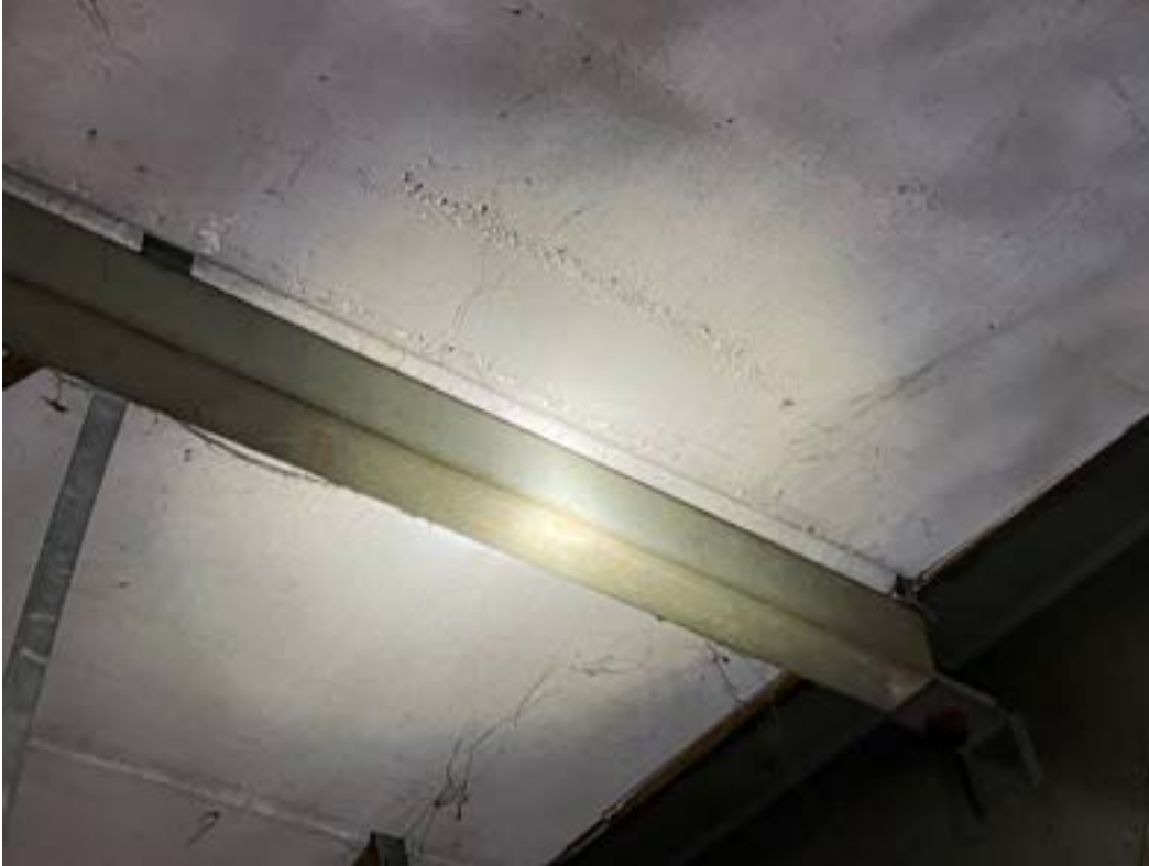
Photograph 18 close up of plank in theatre area with a line of honeycombing and voids. Hairline cracks also in the area but not visible in the photograph.
