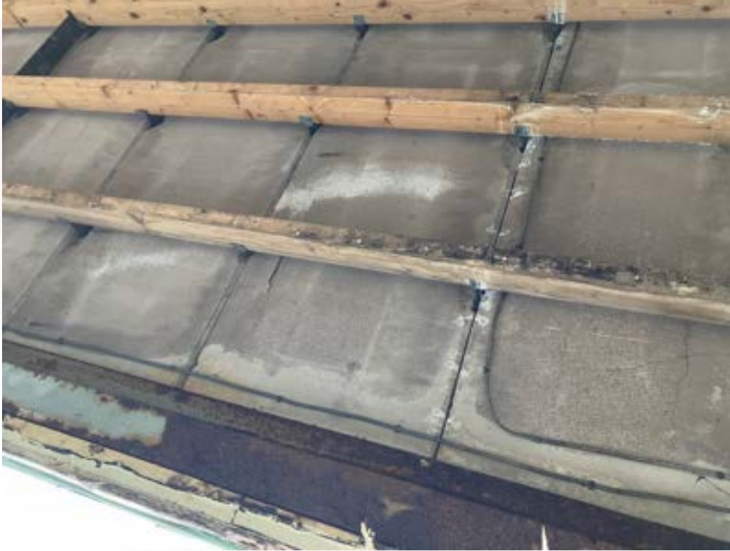
Photograph 11 typical wet panels with damages panels at corners and cracking throughout to walkway area.
