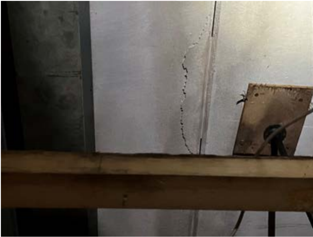
Photograph 15 cracking to panel.
