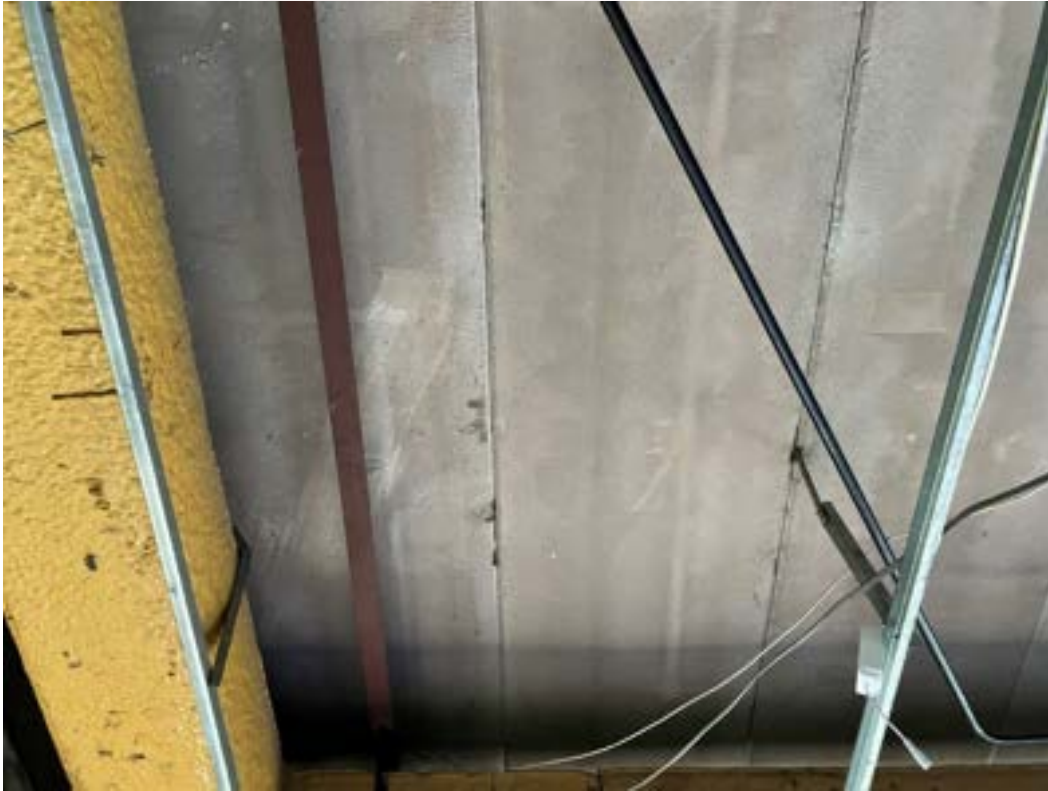
Photograph 9 watermarks to panels, note reinforcement pattern visible.
