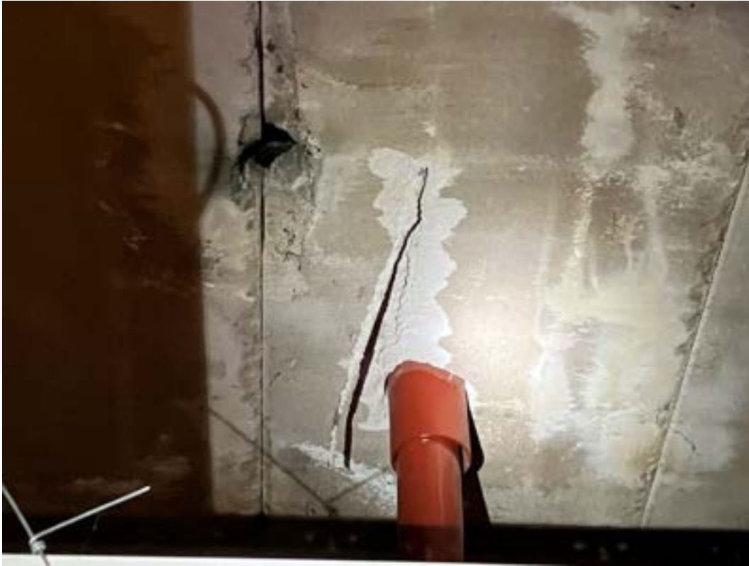
Photograph 8 holes to panels and rebar pulled out of panel for new boiler flue.
