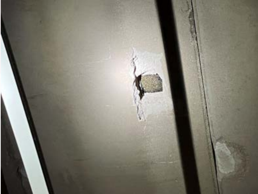
Photograph 3 typical penetration to the slab and further damage in the panel
