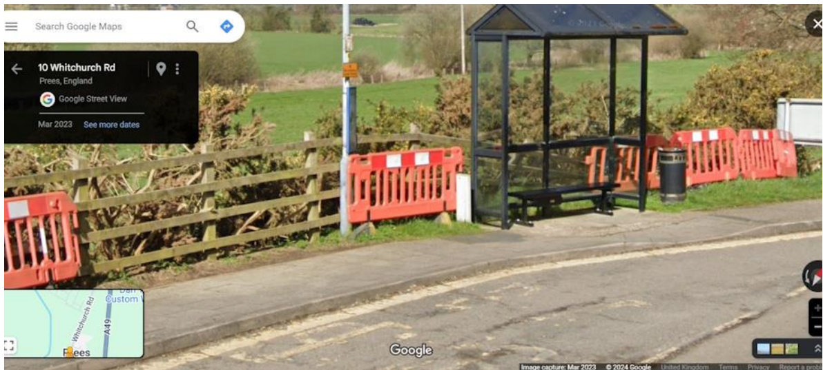
Figure 3 – Recent instability on the highway embankment (see emergency fencing, area of falling fence behind bus shelter and re-patching of tarmac).
