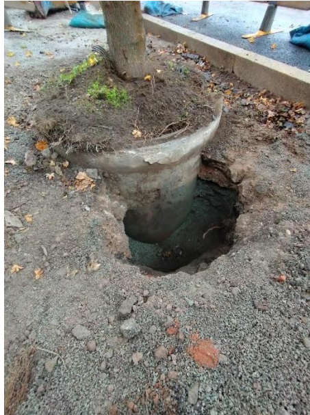
Figure 4-1 – T4 located in 1200mm wide x 1000mm deep concrete ring underlying recently removed tree pit and hard surface.
